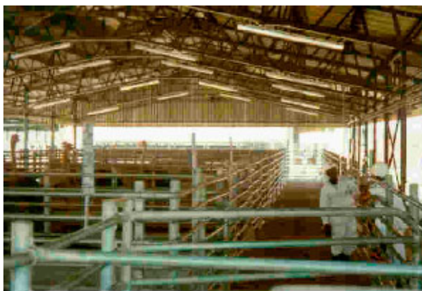
Fig. 21: Smooth tubular rails for pen partitions
